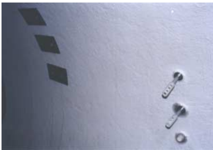
Fig. 6. View of corrosion coupons (3 pieces), ER probes (2 pieces) and reference electrode mounted on the internal surface of water pipeline
